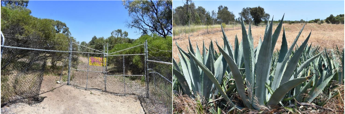
Damaged fence at Mandurah Rd Entrance
